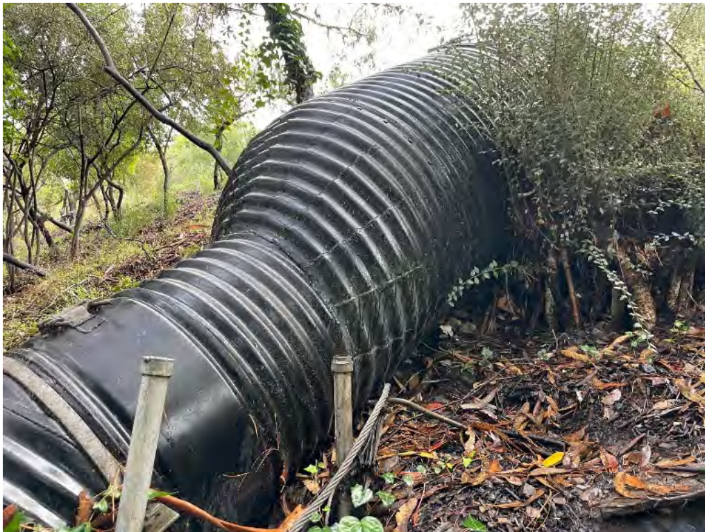
Figure 6. Storm drain carrying Willow Creek flows on the north (downstream) US 101 embankment, reducing pipe size from 48 inch to 30 inch diameter.
