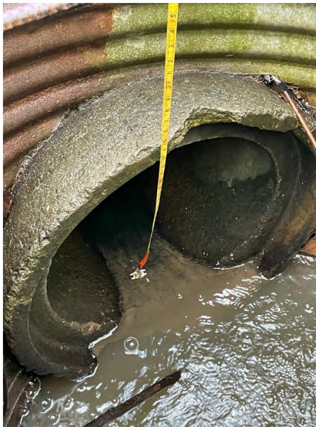
Figure 8. 24-inch diameter storm drain inlet at Lincoln Drive conveying Willow Creek flows through the school campus to Buchanan Drive.
